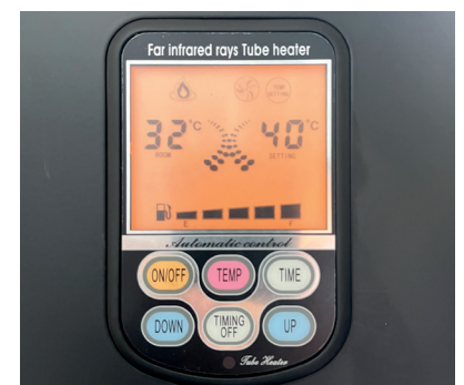
Digital display with control panel
